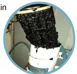
Diesel "bug" microbial contamination creates a slime called a biofilm or biomass
