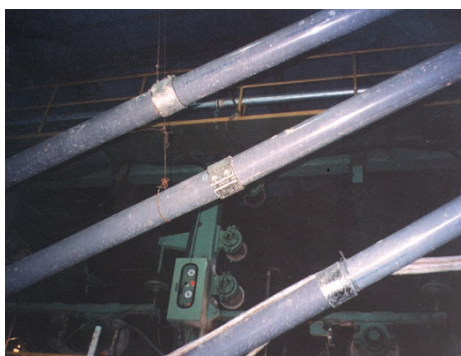
MJS EPDM 200A. pulp conveying line. PVC pipe. couplings used for pipe connection for pipes to be cleaned regularly. Korea
