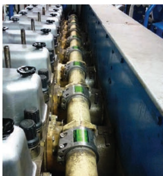
MJG EPDM 100A. engine room. Australia
