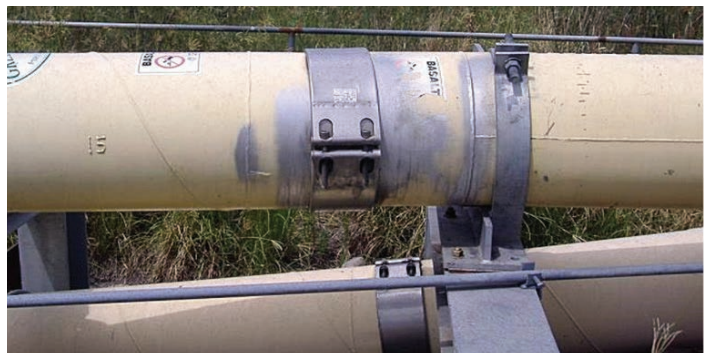
MJS EPDM 400A. mineral conveying line. Australia
