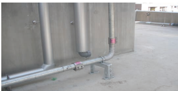
MJGF EPDM 50A. fire protection system. Japan
