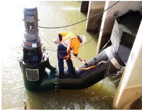
MJS EPDM 600A. hydroelectric plant. Australia
