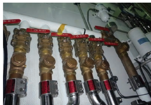
MJG NBR 40A. engine room. Taiwan
