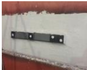
Anode after service 维修更换后的阳极
